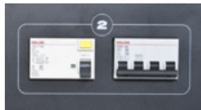
RESIDUAL CURRENT DEVICE (RCD) / 4 POLE CIRCUIT BREAKERS FOR EACH DIMMER
