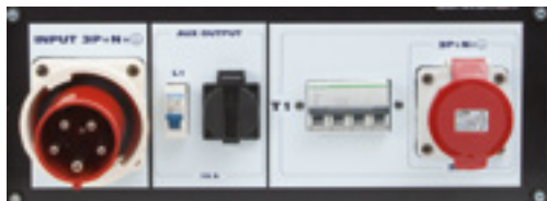
Three-phase connector (3P+N+E) of 63 A. Two additional outputs (32 A three-phase 3P+N+E and 16 A schuko mono-phase) with their own circuit breaker.
